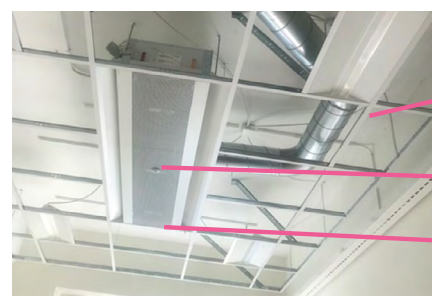
Figure 9: Smart system components: The intelligent building control includes sensors, lighting, and the chilled beam which allows control temperature and ventilation.
