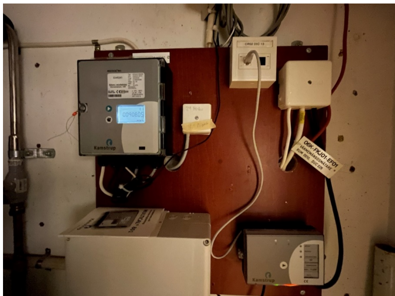
Figure 19: The energy meter that registers the amount of cooling being traded.
