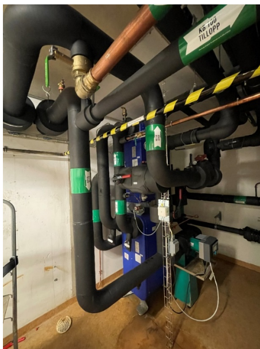
Figure 20: The connection point between the VCC cooling grid and the UEAB cooling grid.
